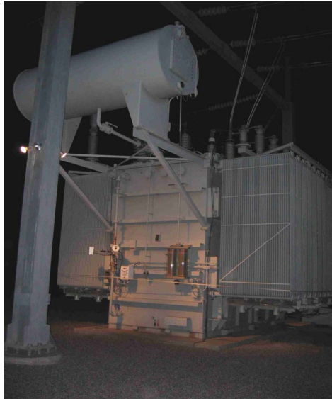
Fig. 5 – Photograph of one of the two 250 MVA transformers tested
